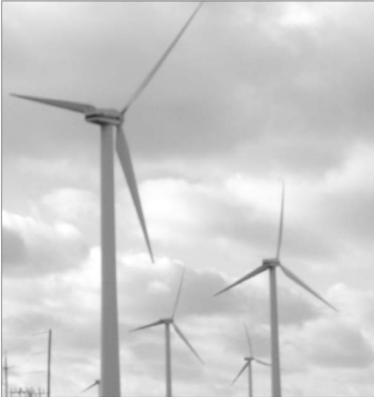
The wind mills at the test site in North Cape, Tignish were working hard Dec. 2 with winds gusting up to 78 km/h.
