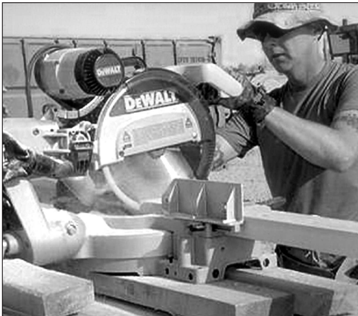
Montague native Corporal Shane Llewellyn saws wood to be used in the construction of a new Canada House at the Kandahar Airfield in Afghanistan. Llewellyn was one of the 40 Canadian engineers sent to the airfield to construct a variety of projects. Submitted photo.
